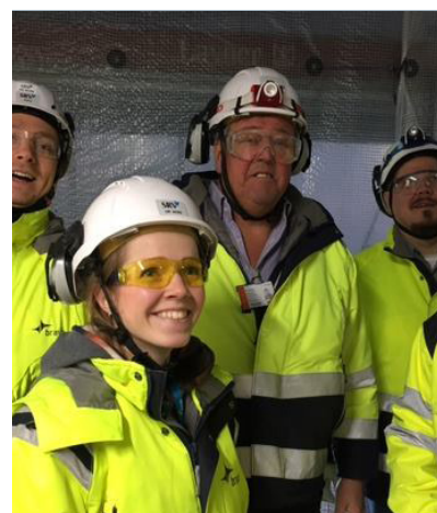
In Finland, Bravida is installing heating & plumbing and HVAC fittings for a project in Espoo
